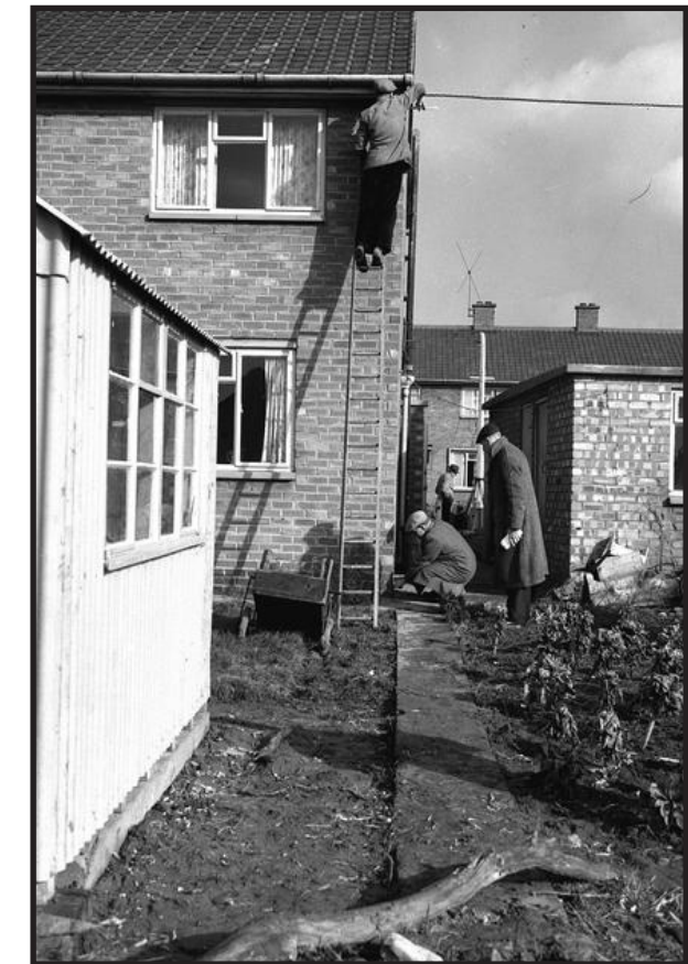
Work to the rear of a house in Thoresby Road, 1956 - City of York Archives
