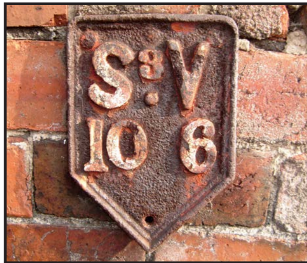
Sluice valve marker on Murray Street
