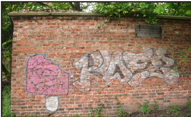
Boundary wall facing south onto the moor featuring a commemorative plaque regarding Quaker Burial Ground and graffiti.
