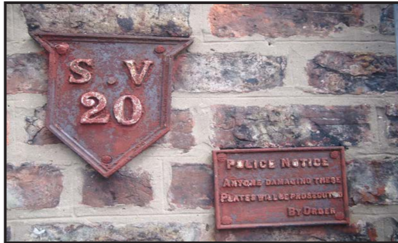
Sluice valve indicator and police notice ('anyone damaging these plates will be prosecuted') on Ruby Street.
