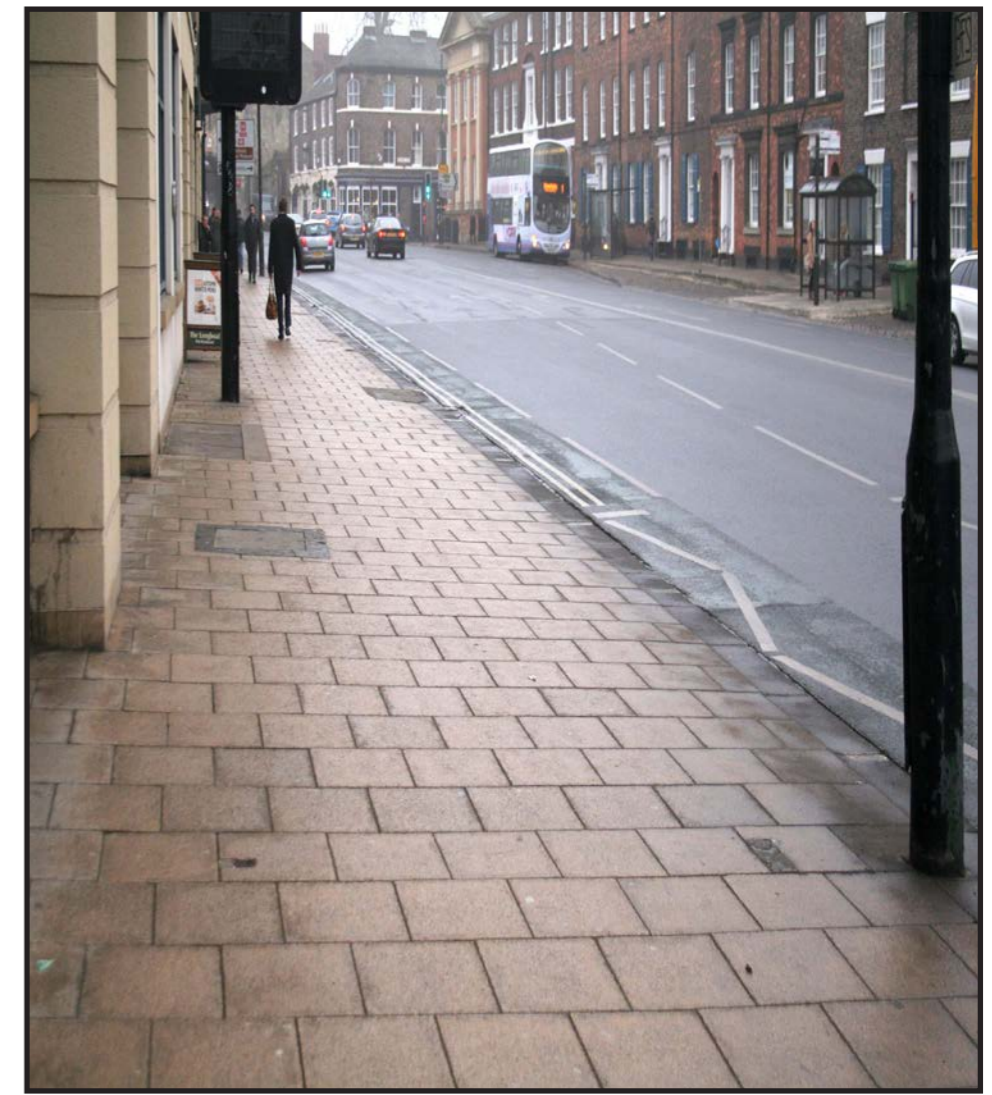
A large area of 450mm x 450mm Saxon paving on Blossom Street. Use of 900mm x 600mm sized flags in conservation grey would be more in keeping with the scale and importance of this gateway street
