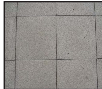
Grey Marshall's Perfecta paving on Lendal Bridge laid as a stacked bond
