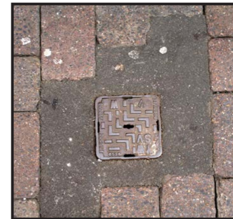
An extremely poor example of repair work by utility contractors using cement rather than the original brick paviments
