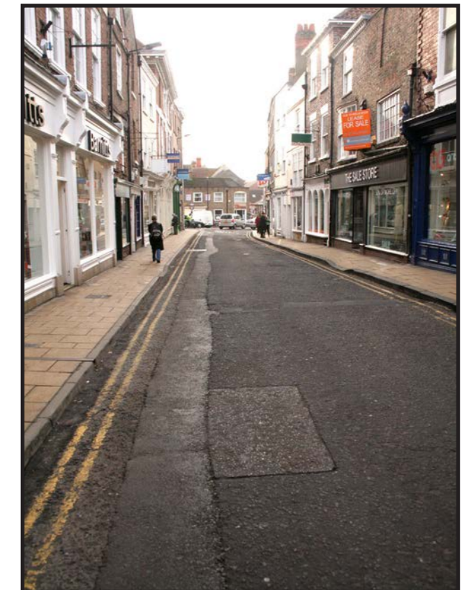
Colliergate with narrow footways badly surfaced in small square pre-cast Saxon flagstones and a poor quality carriageway surface
