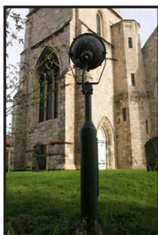
An elderly floodlight with a high pressure sodium luminaire aimed at the tower of St Deny's Church, Walmgate
