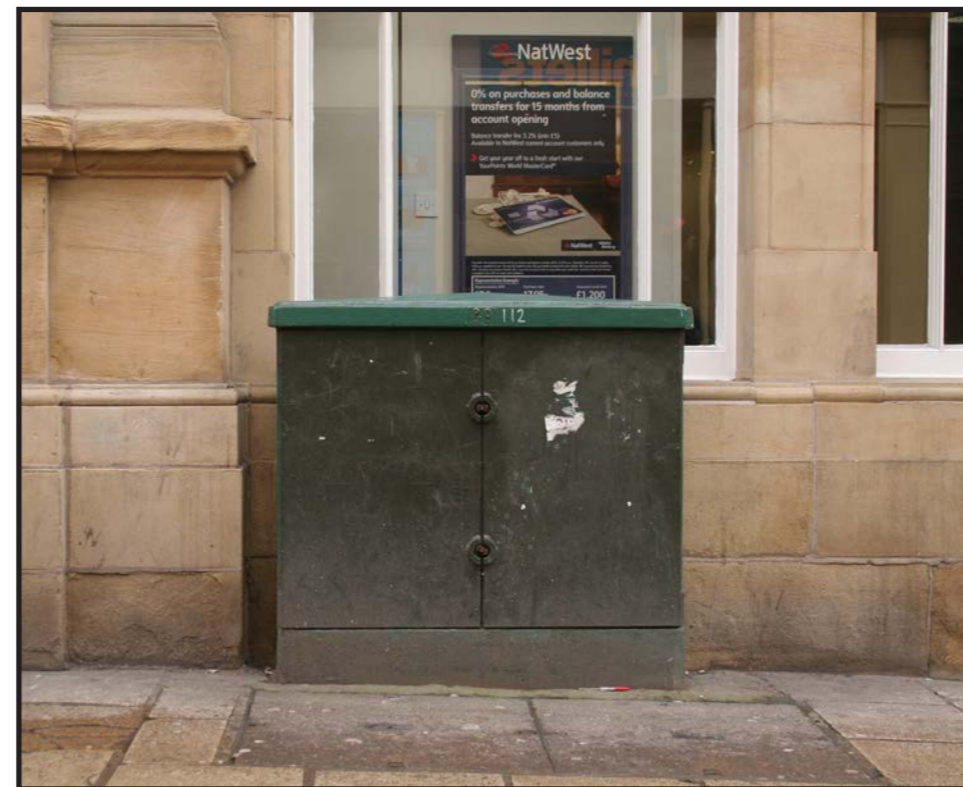
Green cabinet contrasting poorly with warm Magnesian limestone on Market Street in the centre of the footstreets. Gloss black would improve this although relocation would be preferable, where technology changes.
