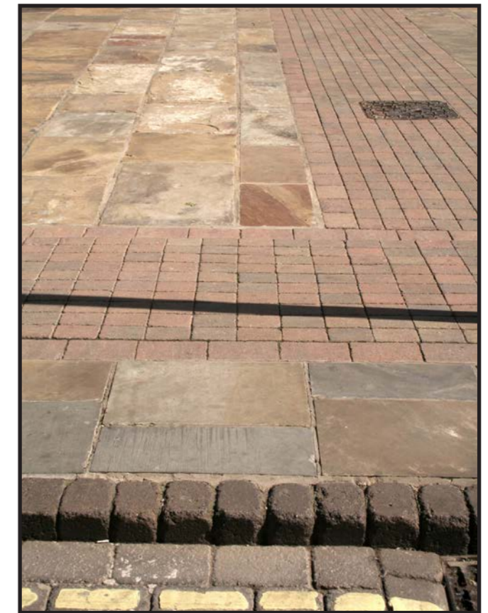
Mixed natural and manufactured materials on Parliament Street, resulting in a poorly designed and over complex public space
