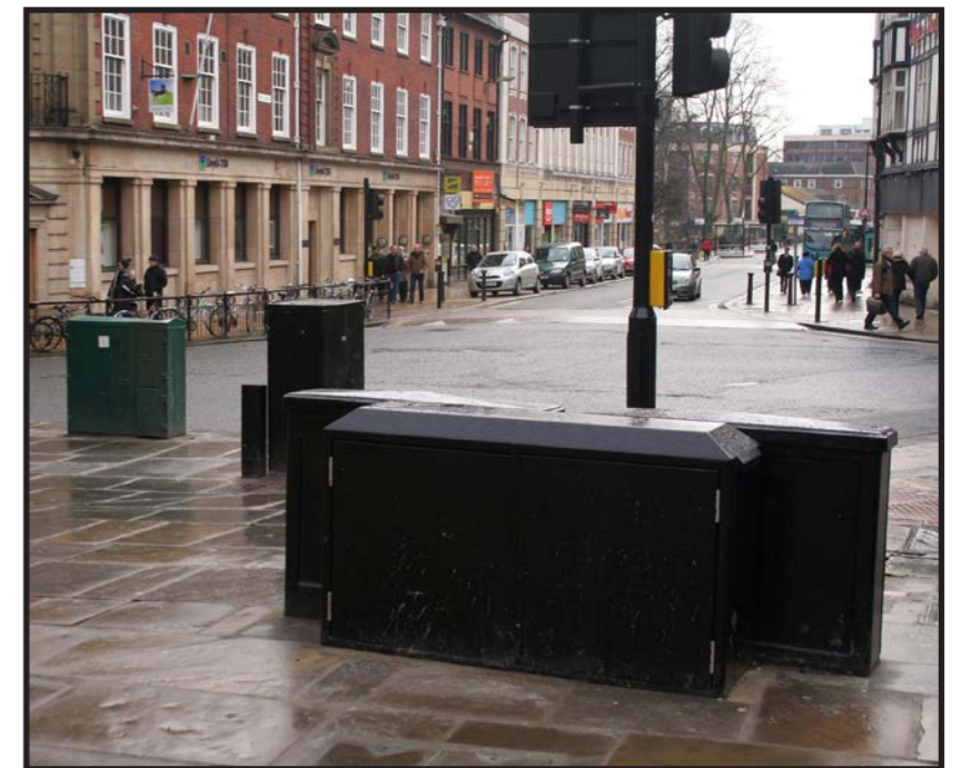
An unfortunate collection of cabinets in black and green at the junction of Parliament Street, Pavement and Piccadilly. Opportunities to rationalise this situation should be taken with utility companies and the Council's Network Management function.
