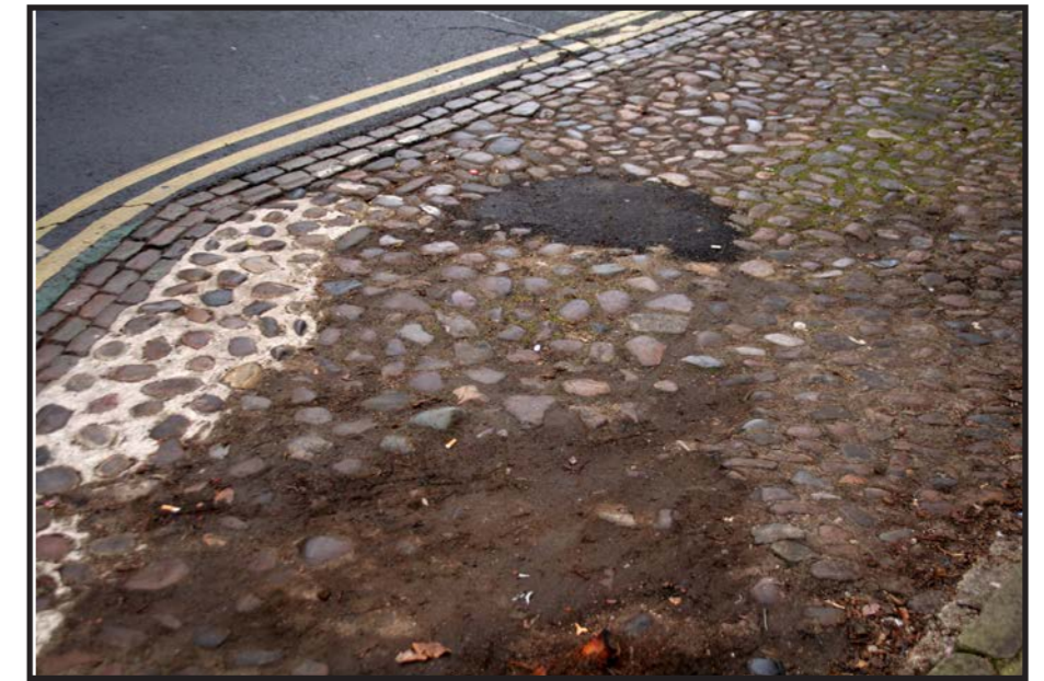
Cobbles on Blossom Street with contrasting reinstatement (white cement) and repair (asphalt) resulting in a significant visual detractor on this historic gateway street. The spacing of reinstated cobbles is also poor.
