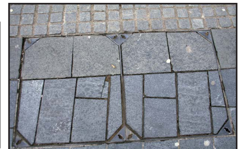
A poor example from Sheffield where more than one material has been used to infill the inspection cover
