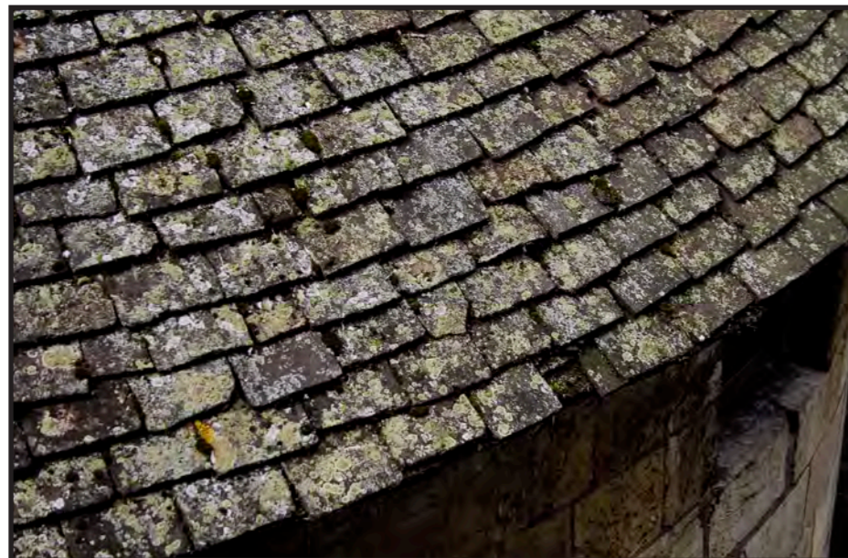
14th century Barker Tower with magnesium limestone ashlar and English Pennine Sandstone roof tile.
