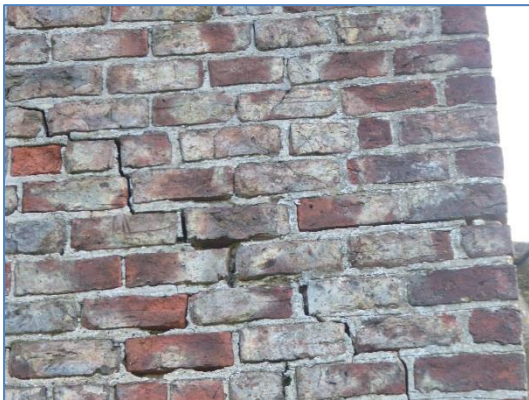
Photo 25: Building 3 crack in external wall
