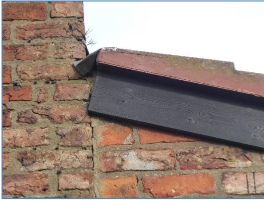
Photo 21: crevice on southern aspect, on edge of extension
