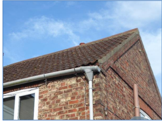
Photo 22: lifted tiles at eaves on farmhouse
