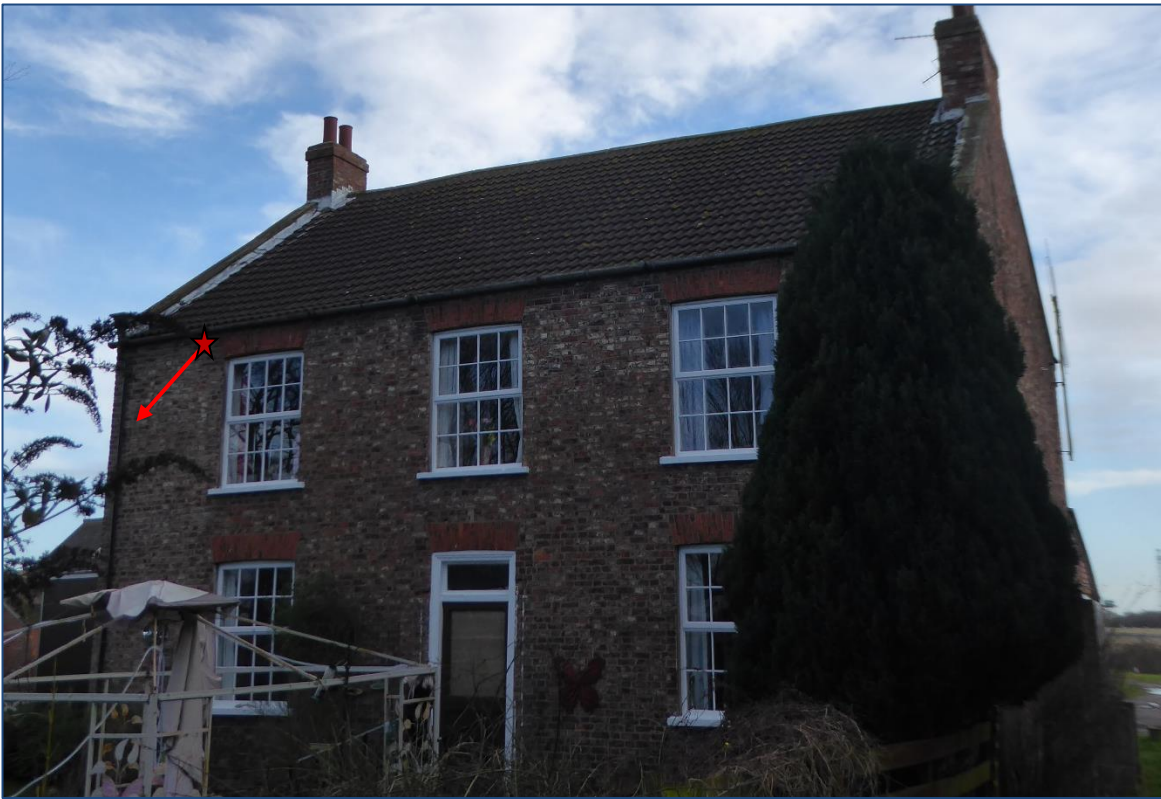
Photo 57: Building 1; masonry crevice under guttering by north west window
