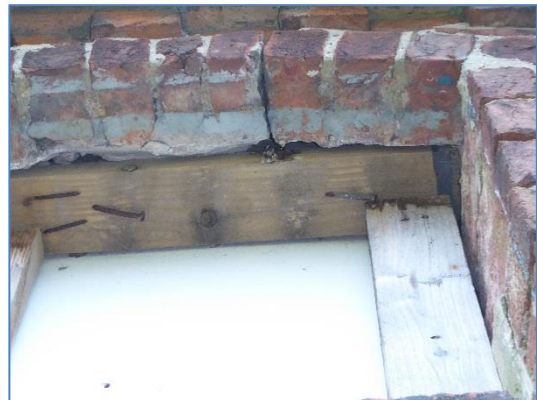
Photo 26: Building 3 crevices in window lintel
