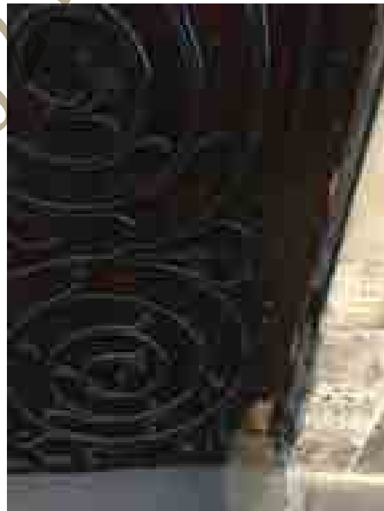
Fig. 45: Damage to historic doors
