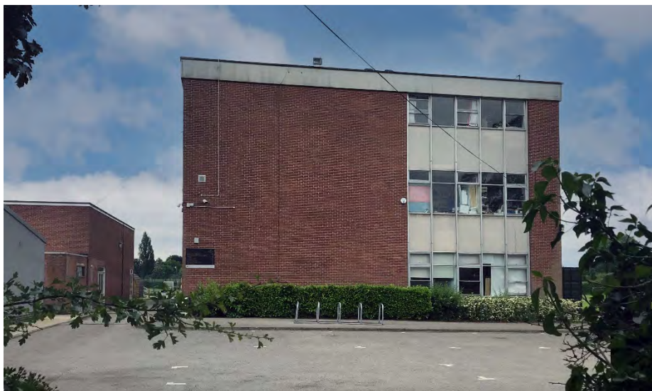
Poor quality CLASP procured previous LA stock in need of replacement has minimal architectural value in terms of fenestration and quality of build.
