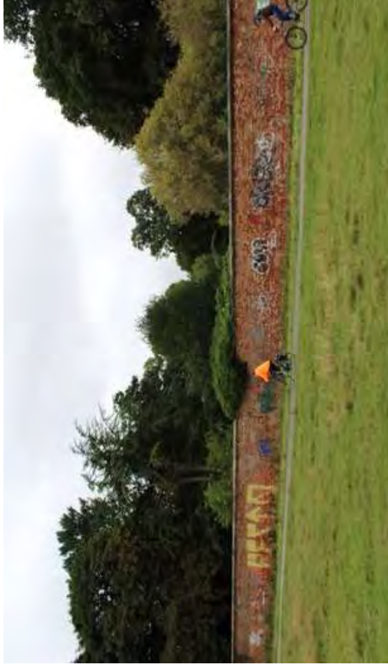
▲ D. High brick boundary wall running along southern boundary adjacent to Walmgate Stray.
