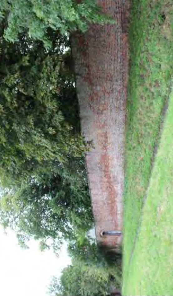
▲ C. High brick boundary wall running along western boundary adjacent to Walmgate Stray.
