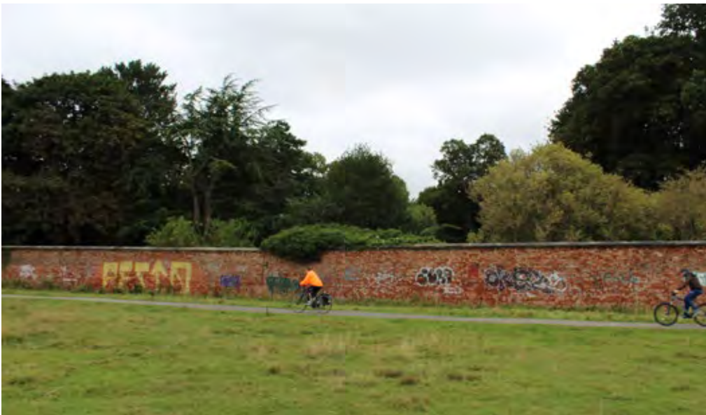
▲ D. High brick boundary wall running along southern boundary adjacent to Walmgate Stray.
