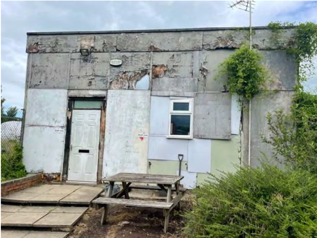
An auxiliary building at the north of the site in poor condition category D
