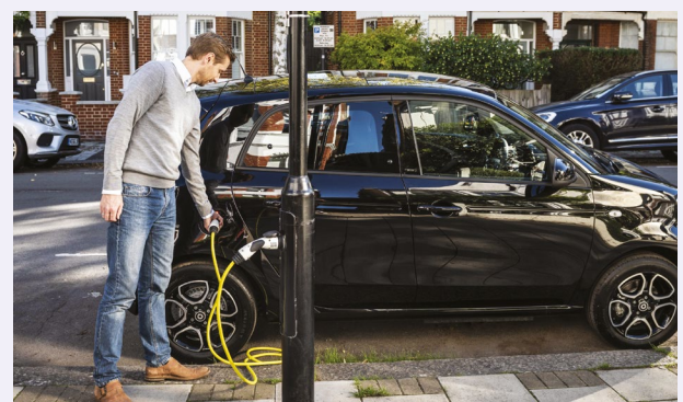
Figure 9K - Lamp post charging point. Credit: Ubitricity/Shell
