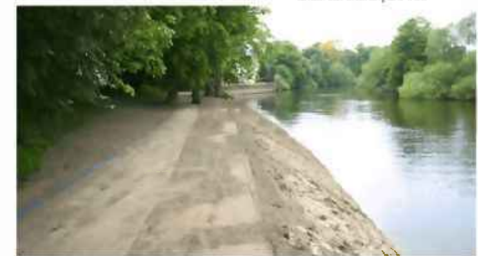
2002 new riverside walk constructed over rockfill and gabions (approximate extent of lost burial ground)
