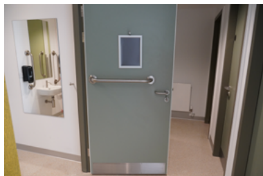
Horizontal rail to the back of the door is too high.
