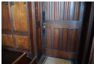
Door handle in the corner with obstructed access to it.
