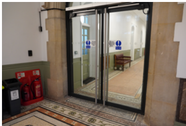
The proximity reader is located within the door swing.
